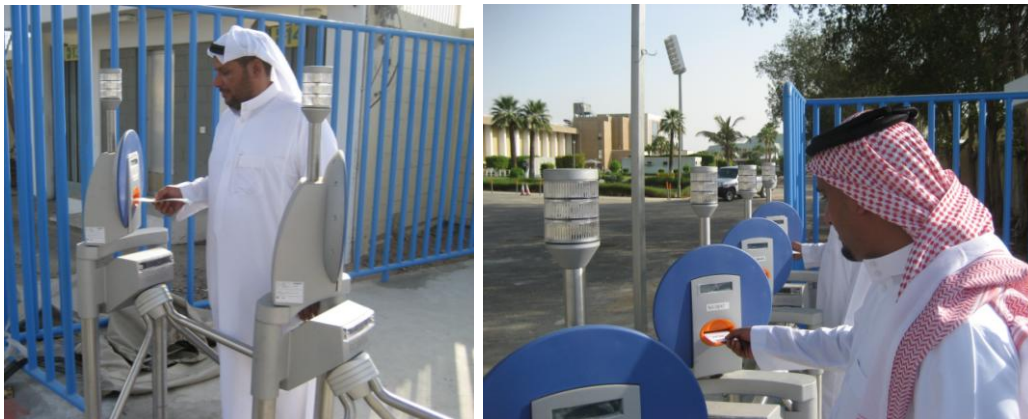
Access Control System – Jeddah Stadium
